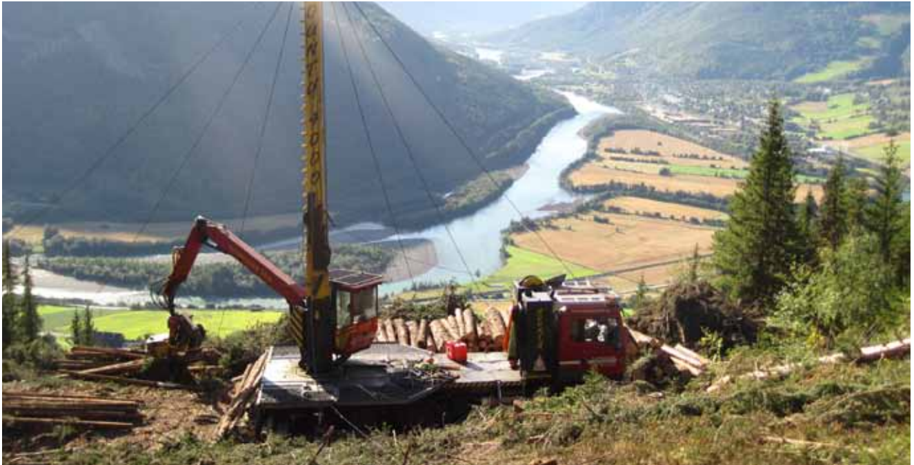
Cable-yarding in steep terrain is an example of the variable conditions for harvesting operations in the Nordic countries. The OSCAR conference took a narrow look at the method. Of special interest were the full scale Konrad 'Mounty' 4000' yarder-processor, operated by Frivik Taubanedrift AS, and the new 1:3 scale Owren mini 400 yarder, which was built in Norway for training and recruitment purposes. Photo: Bruce Talbot
